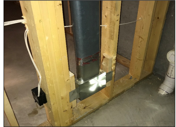
10. Ducted and sealed return air.
