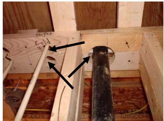
4. Seal all penetrations through the top sill plate on walls. (missing in photo)
