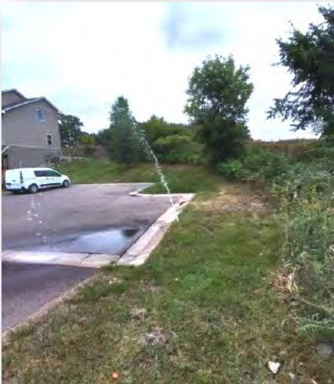
(Above) Due to the nature of irrigation systems running during late night or early morning hours, system breakages like the one seen above are often left unaddressed. Breakages contribute to substantial potable water loss that is easily preventable.
