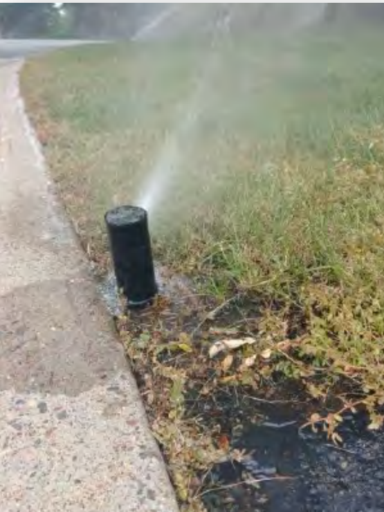
(Above) The sprinkler above, found during one of the HOA system assessments, was estimated to waste half of a gallon of water per minute.
